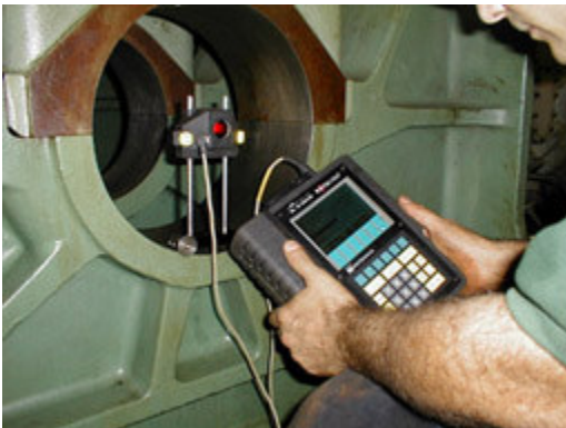
Crankcase Bore Alignment of a Reciprocating Compressor
